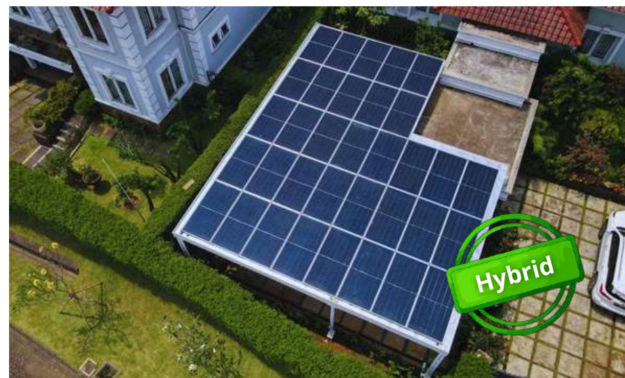
Bogor, Jawa Barat Capacity: 19.89 kWp
