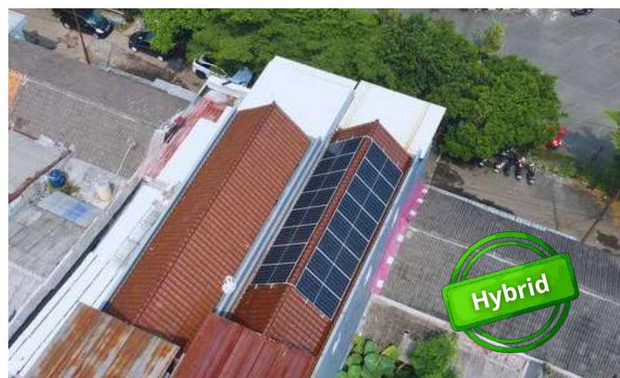
Bogor, Jawa Barat Capacity: 10.32 kWp
