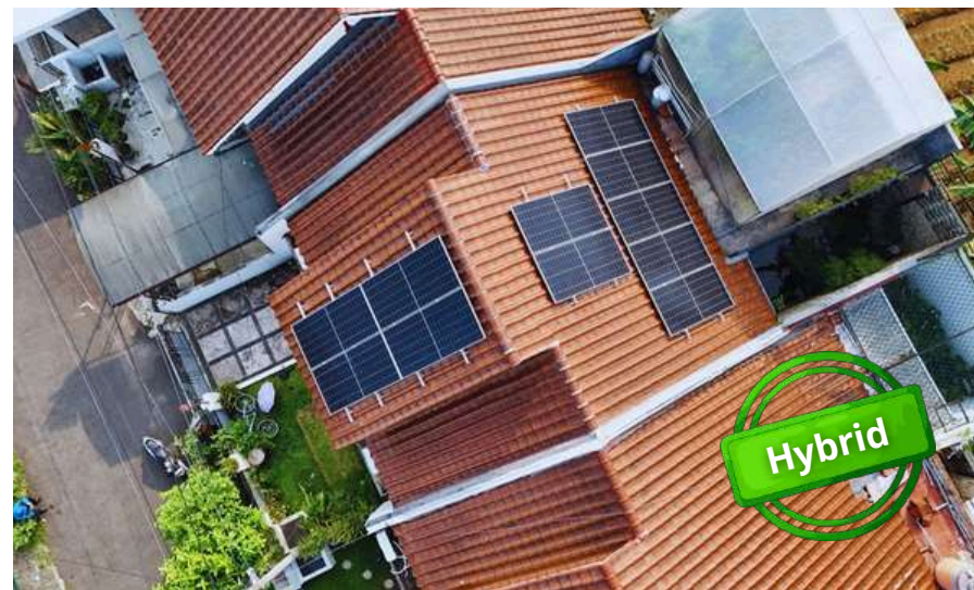
Bogor, Jawa Barat Capacity: 7.095 kWp
