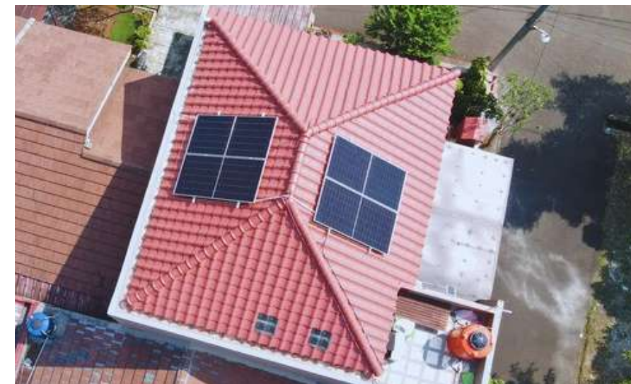
Bogor, Jawa Barat Capacity: 2.6 kWp
