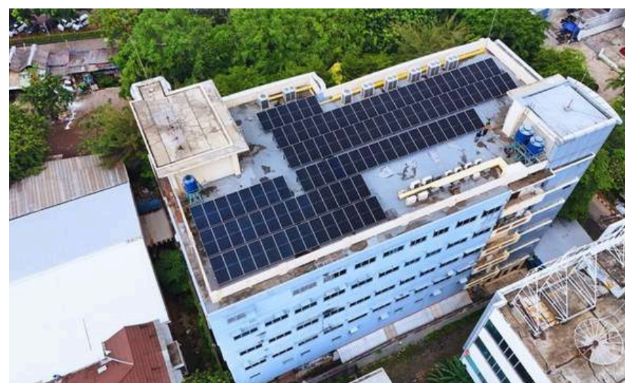
Jakarta Capacity: 69.12 kWp
