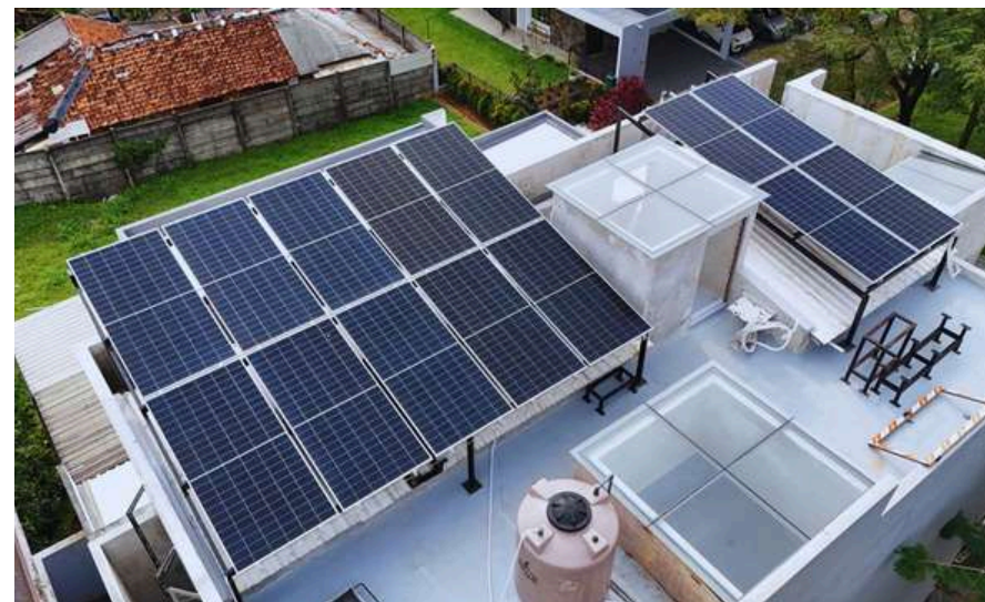
Tangerang Capacity: 8.648 kWp
