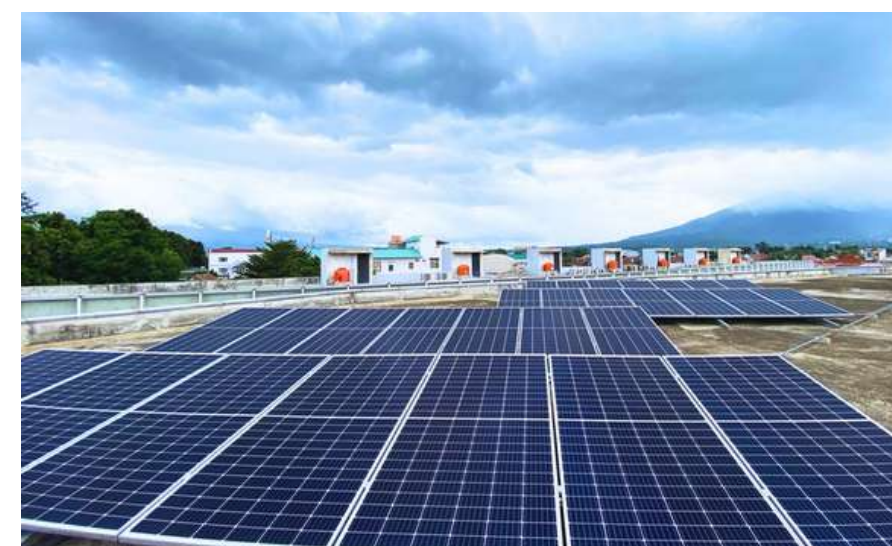
Bogor, Jawa Barat Capacity: 27.73 kWp
