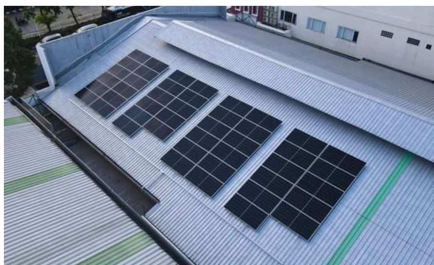
Jakarta Capacity: 28.52 kWp
