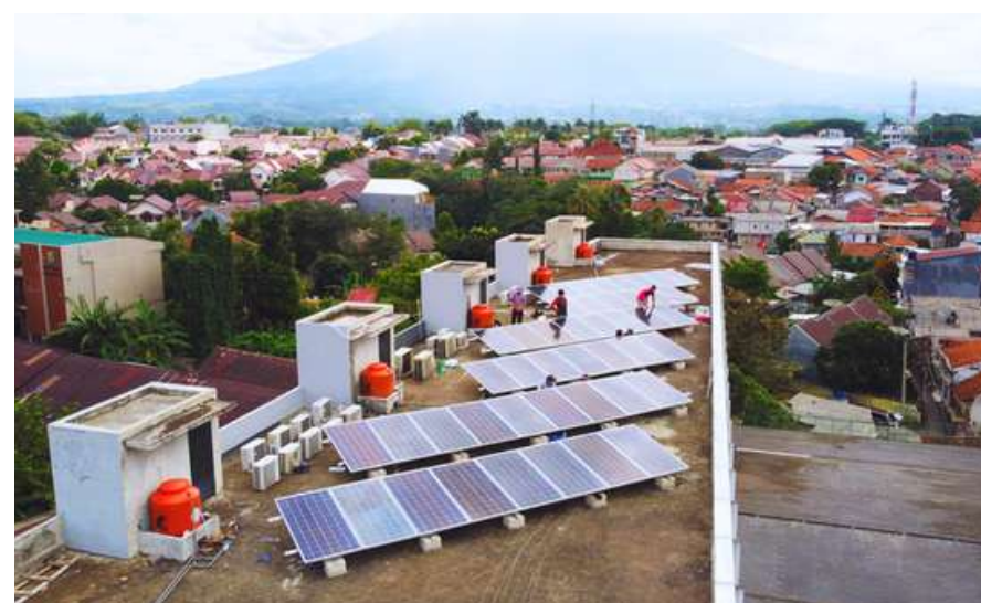
Bogor, Jawa Barat Capacity: 17.02 kWp
